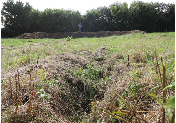
Bund sited in field corner, designed to intercept run-off, holding back water and letting sediment settle before reaching the watercourse
